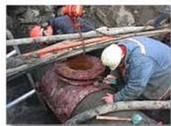
Distribution Crew at work making a repair to a 24 inch water main
