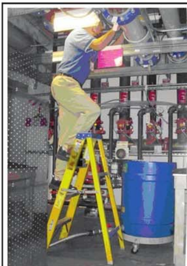
Figure 6. Example of a more difficult place to get UPW samples.
