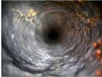
Corrosion of Stainless Steel
